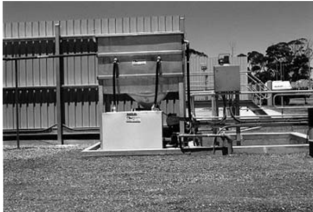
Figure 17.5 Above ground Coalescing Plate Separator, heavy vehicle washpad, Western Australia.
