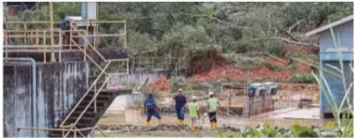
Workers at an Indah Water Konsortium waste treatment plant observing damage to the premises due to a landslide in Taman Wawasan, Puchong, on Dec 16. PIC BY AZUDDIN SAAD
