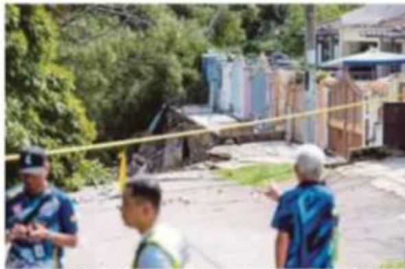
The site of a landslide at Jalan Wawasan, Puchong, on Dec 16 last year. PIC BY ASWADI ALIAS
