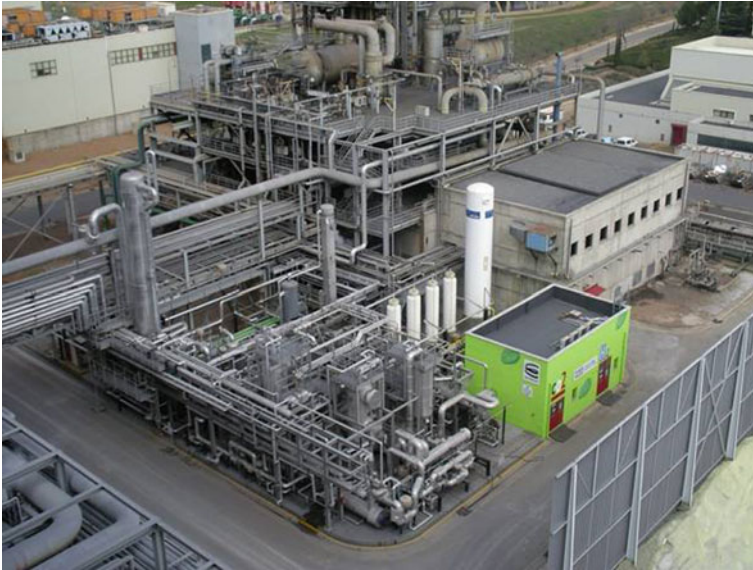
Fig. 7 CO 2 capture and H 2 co-production pilot plant: location
