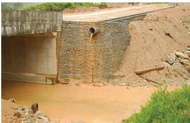
Siltation in river
