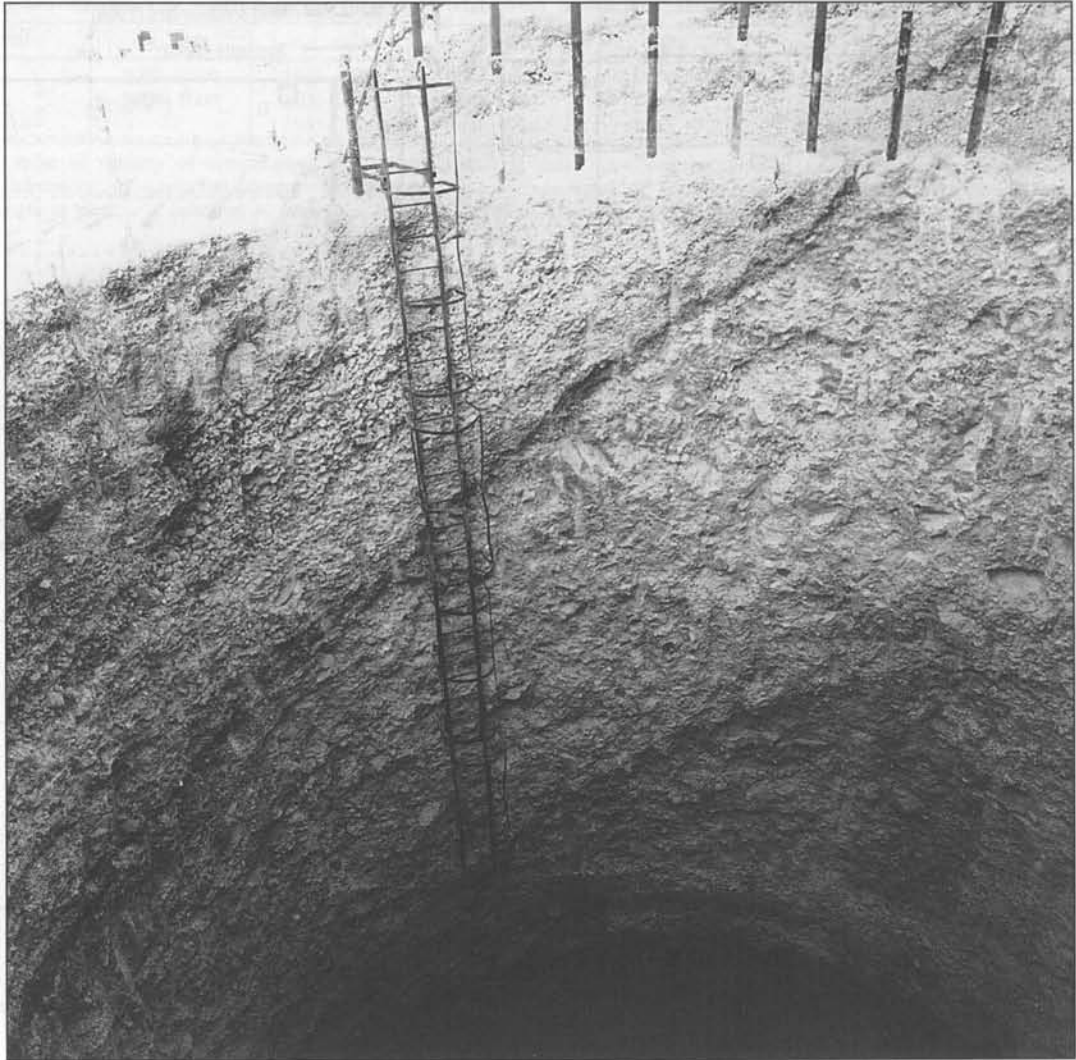
Fig. 11. Shaft wall made of overlapped jet columns (case A), showing the persistent natural soil structure (inclined strata parallel to slope)
