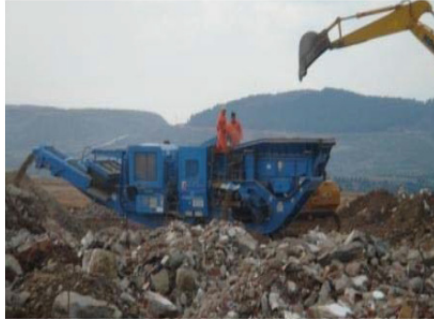
Figure 3. Demolition Waste Recycle Facility [35]
