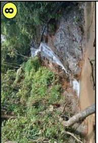
8 Tributary of Sg. Simin in the western portion of the Project Site
