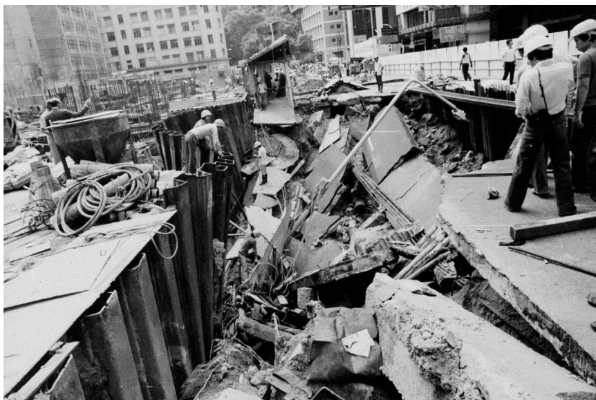
Figure 5.3 Collapse of Queen's Road, Hong Kong 1981.
