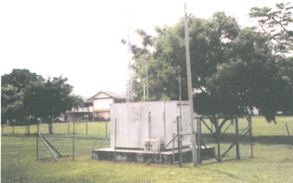
Photo 1: Continuous Air Quality Monitoring Station. (DOE Photo Library)
