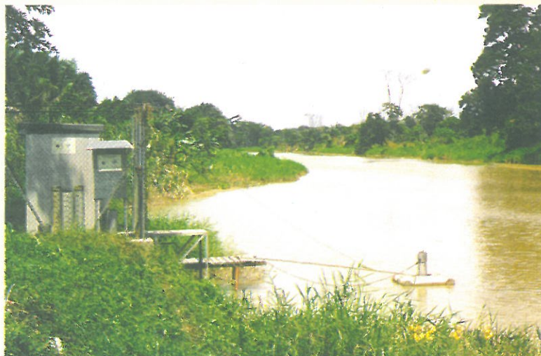
Photo 7: A Continuous Water Quality Monitoring Station (DOE Photo Library)
