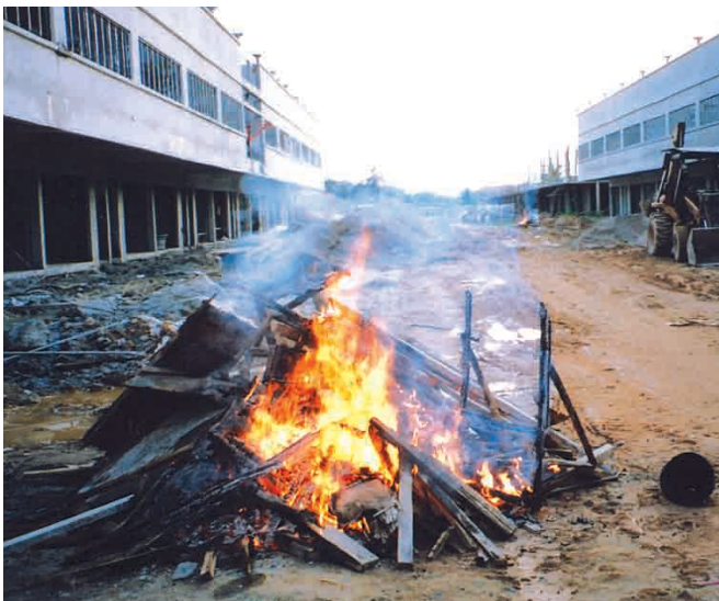
Photo 5: Open Burning at Construction Site (DOE Photo Library)
