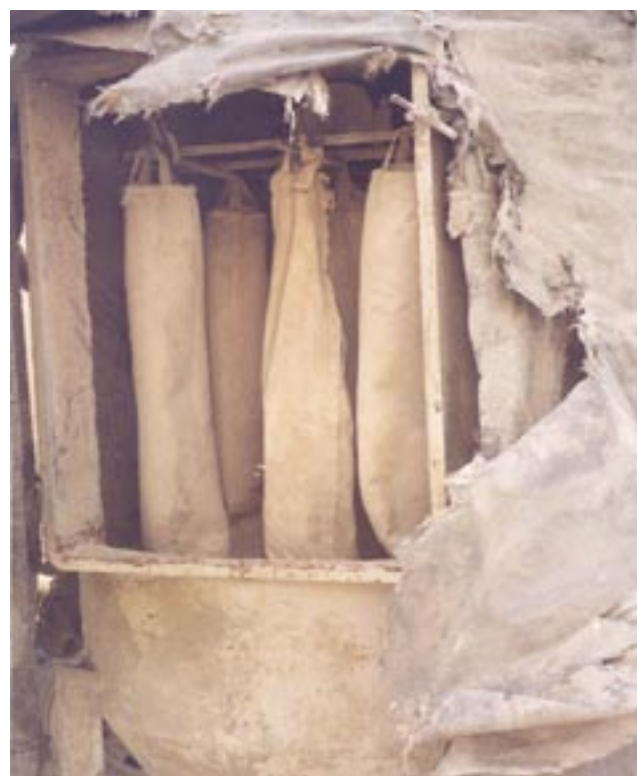
Inefficient Air Pollution (Filter Bag) Control System (DOE Photo Library)
