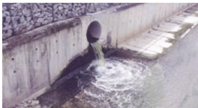
Major Water Pollution Source : Untreated Sewage (DOE Photo Library)
