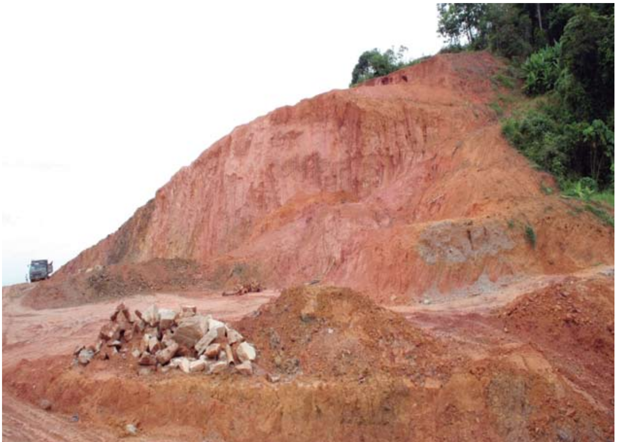
Uncontrolled hill cutting (DOE photo library)
