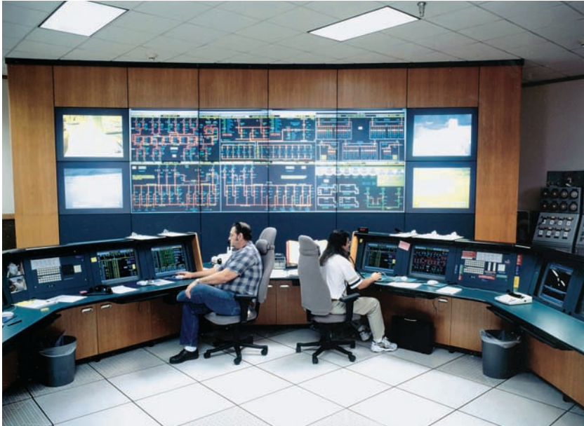
Hoover Dam control room. A small number of people controls one of the nation's great hydroelectric power plants. ( U.S. Department of the Interior, Bureau of Reclamation )
