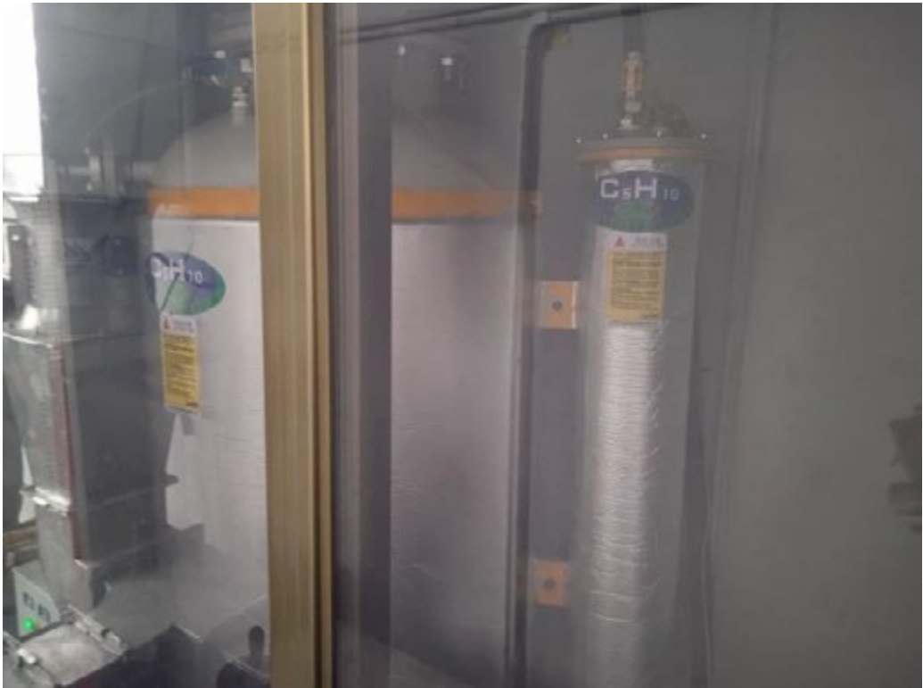
Figure 6.7: Preblended C5 tank is securely installed inside a safety cabinet and equipped with a flammable gas detector
