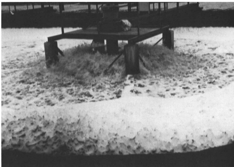
Fig. 7.9. Fixed level surface mechanical aerator in an aerated lagoon.
