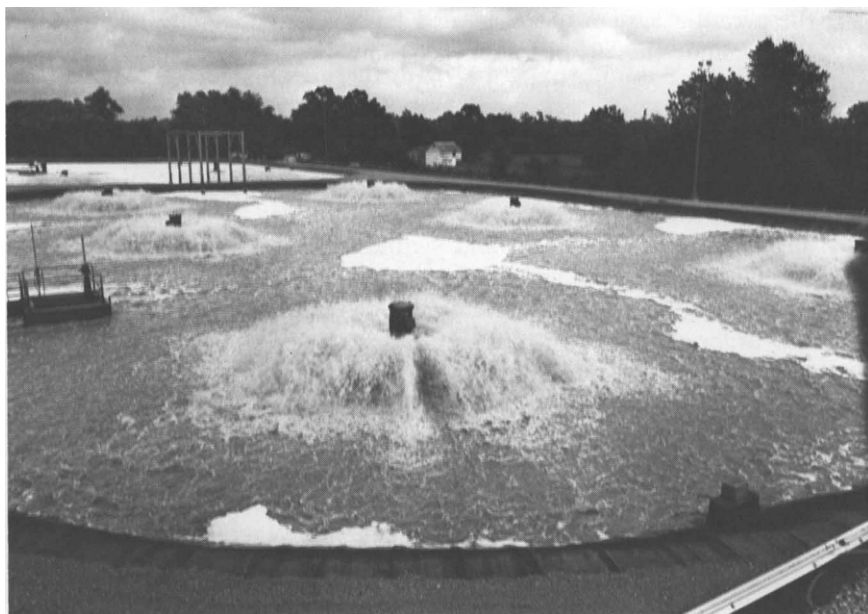
Fig. 6.14. Surface aerators in an aerated lagoon treating brewery wastes (courtesy Rexnord Envirex, Inc.).
