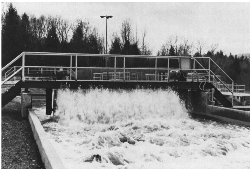
Fig. 7.21. Aeration and turbulence caused by rotors in an oxidation ditch (courtesy of Lakeside Engineering Corp.).
