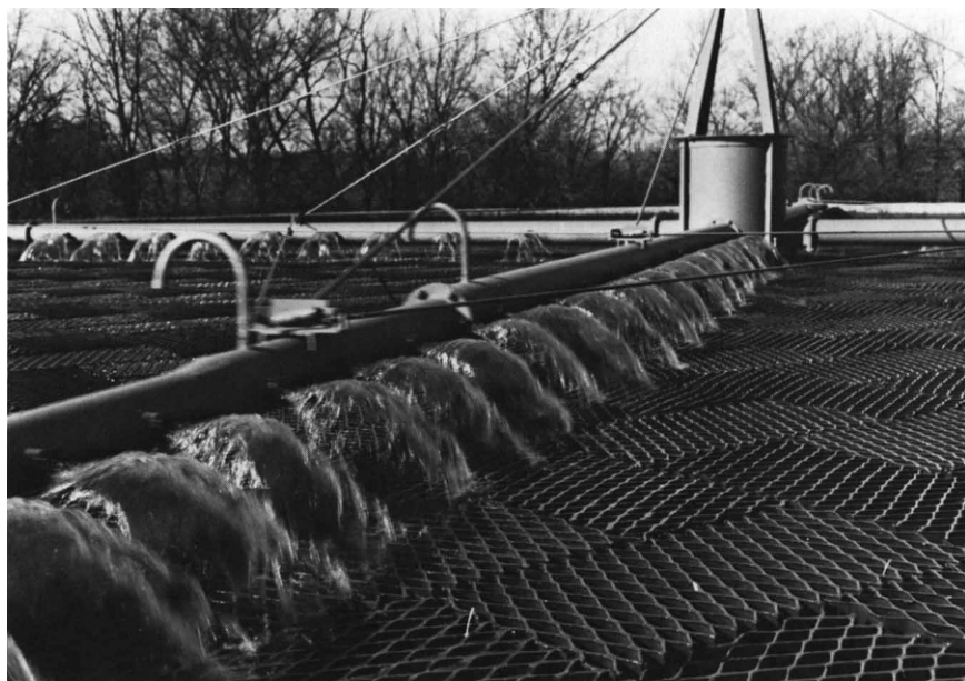
Fig. 7.31. Plastic media trickling filter and rotary distributor (courtesy Dow Chemical Co.).
