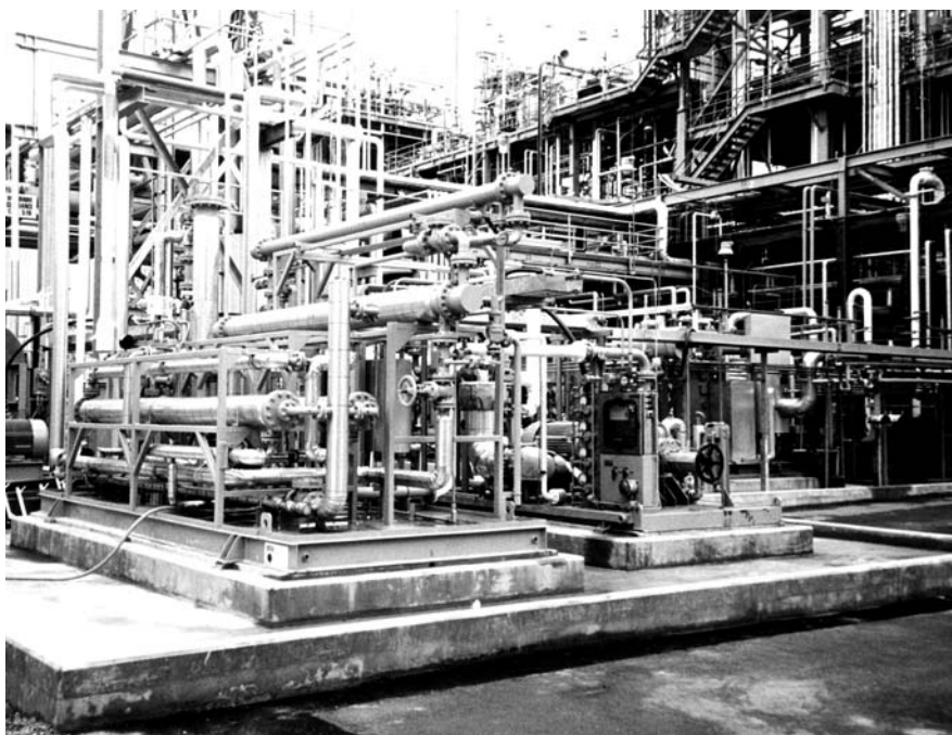
Figure 8.36 Photograph of a membrane unit used to recover nitrogen and propylene from a polypropylene plant vent gas
