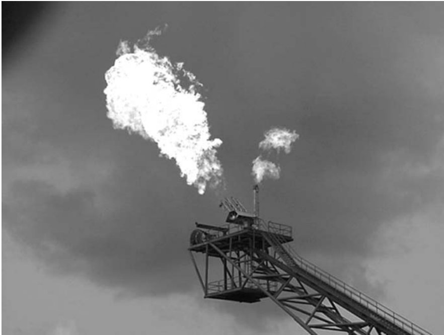
Figure 1.15 Flare on an offshore oil platform without water injection. (Courtesy of John Zink Co., Tulsa, OK.)
