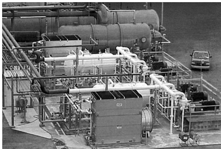
Figure 15.56 Photograph of a flare gas recovery system. (Courtesy of John Zink Co. LLC.)
