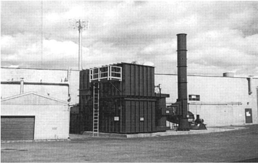
Figure 7.27 Regenerative thermal oxidizer. (Courtesy of Alstom.)
