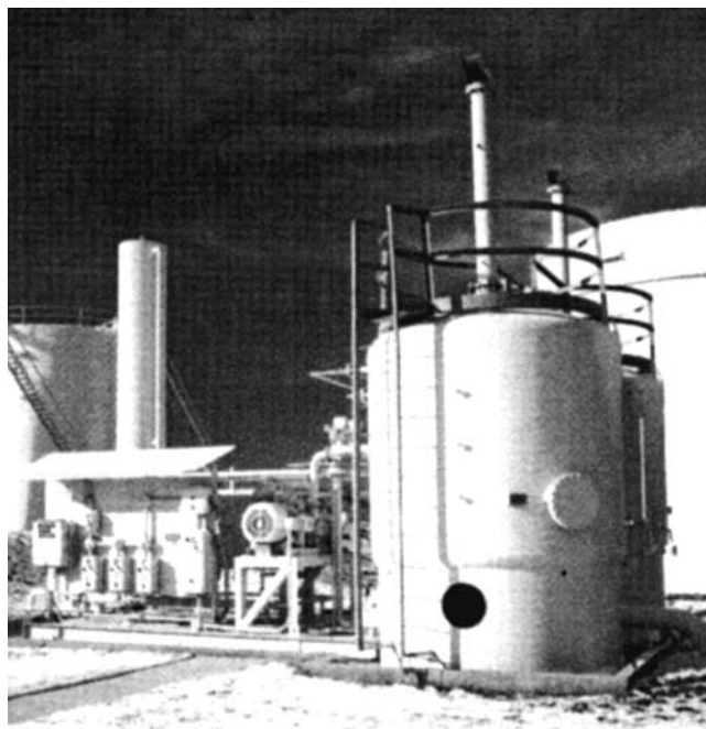
Figure 7.33 Industrial vapor-recovery system. (Courtesy of John Zink Co., Tulsa, OK.)
