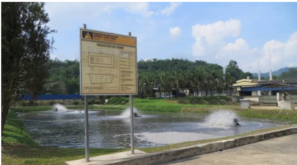
Sistem Pengolahan Effluen (SPE) di Kilang Getah Asli Mentah Effluent Processing System (EPS) in Raw Natural Rubber Factory
