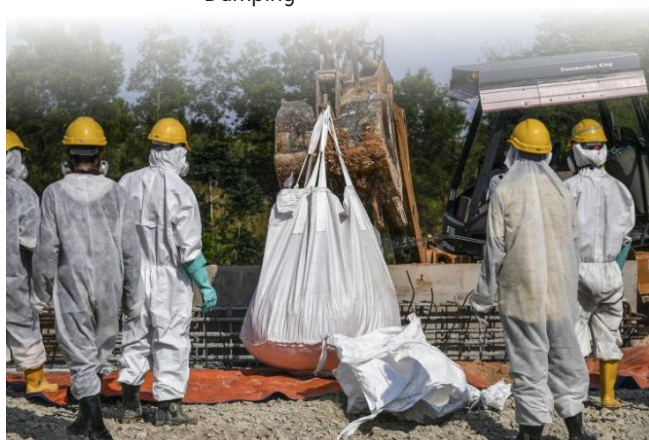
Figure 2.8 Taman Velox, Rawang Chemical Waste Dumping
