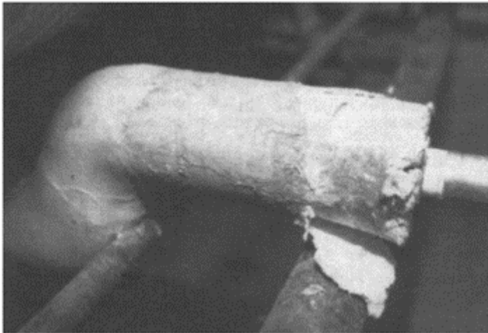
Figure 11.3 Partially damaged asbestos thermal system insulation.
