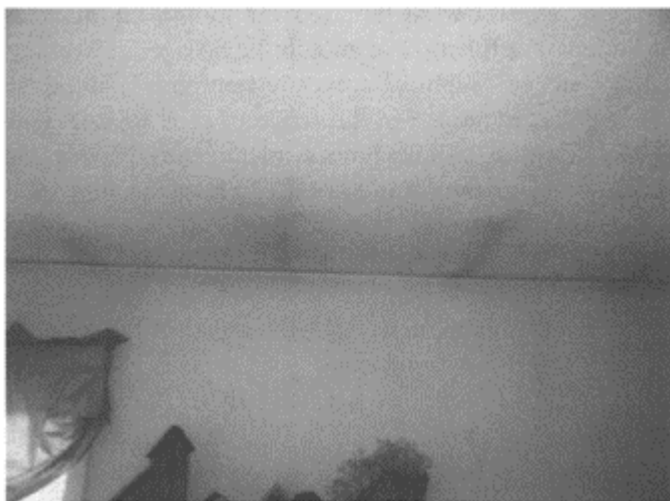
Figure 11.9 Ghosting in a residential building.
