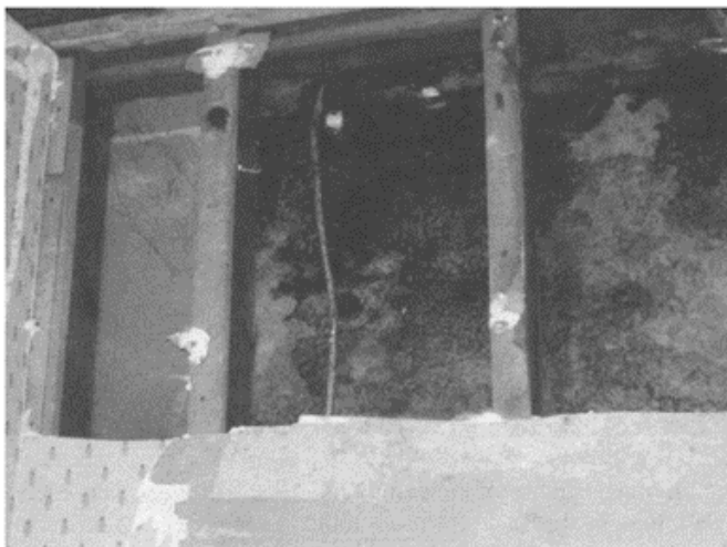
Figure 11.11 Stachybotrys growing on water-damaged gypsum board.
