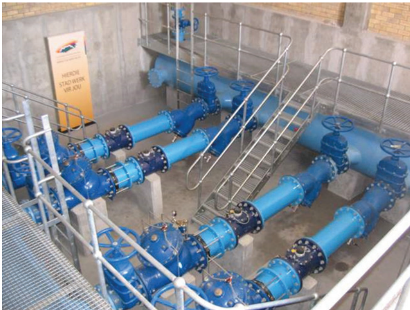
Figure 3.33 Mitchell's Plain pressure management installation.
