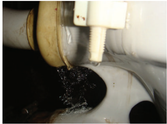
Figure 5.14 Leaking toilet fitting in school.
