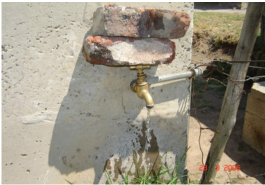
Figure 5.13 Leaking tap in school.
