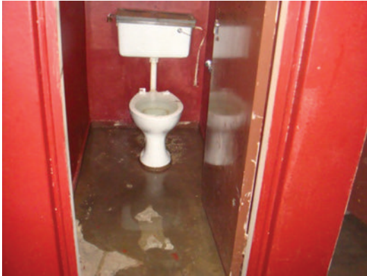
Figure 5.11 Leaking toilet in school.
