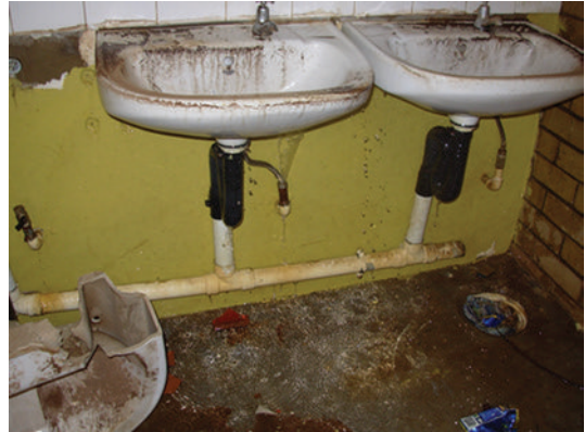
Figure 5.12 Vandalized toilet in school.
