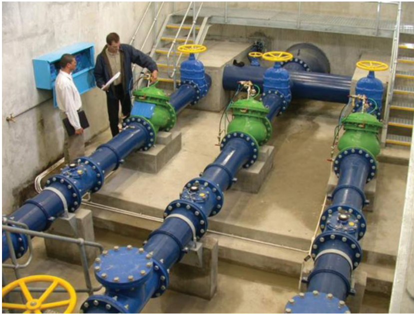
Figure 3.25 Khayelitsha pressure management installation.
