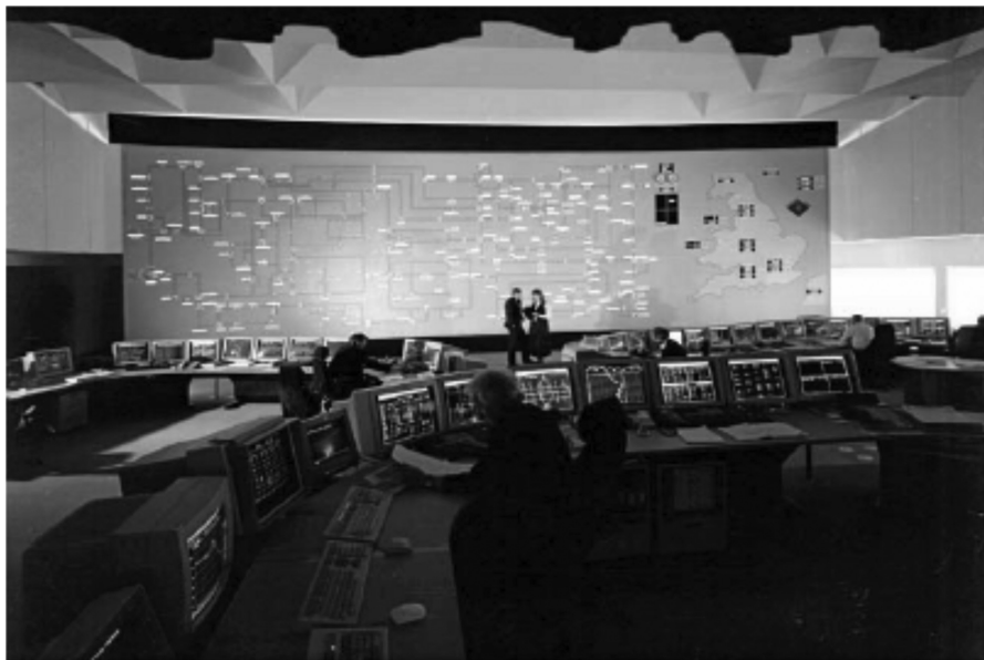
FIGURE 4.3 Central control room.
