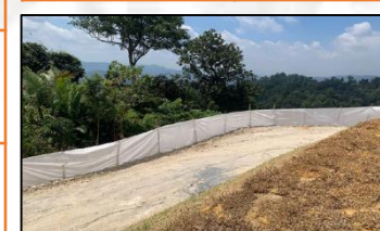
Example of Silt Fence
